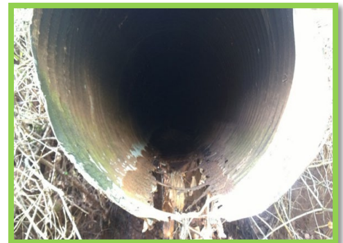
Figure 4. Outfall pipe damage (could indicate the presence of contaminated discharges).
