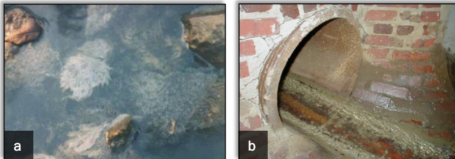
Figure 2 - Sewage. A strong organic or sewage-like odor can indicate a sanitary sewer leak or overflow. Indicators of sewage discharge can include (a) sewage fungus and (b) bacteria growth in outfall.
